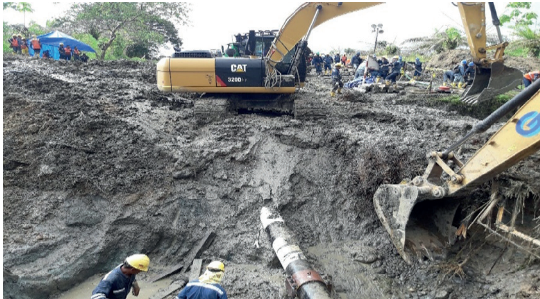
Figure 1. Esmeraldas-Santo Domingo Pipeline Rupture, Ecuador.
